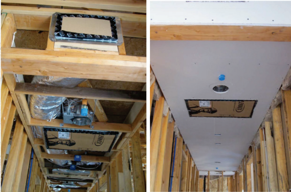
Figure 4-11: Ducts Routed through a Dropped Ceiling
