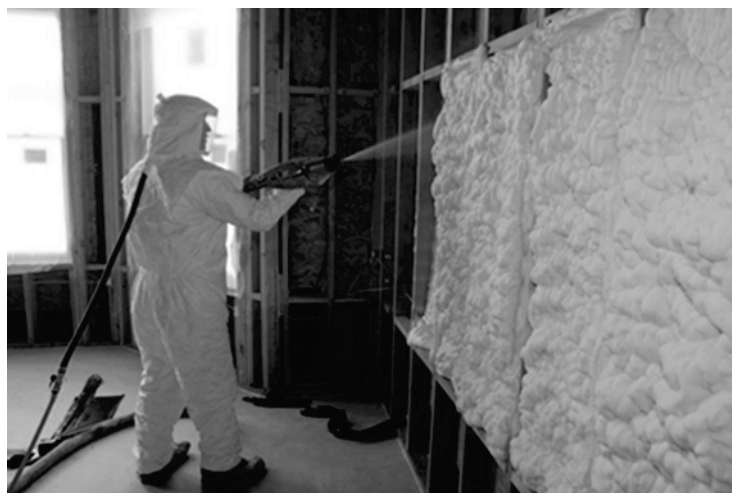
Figure 3-51: Open-Cell SPF Installed in Wall Cavity (may be trimmed to facilitate interior cladding installation)
