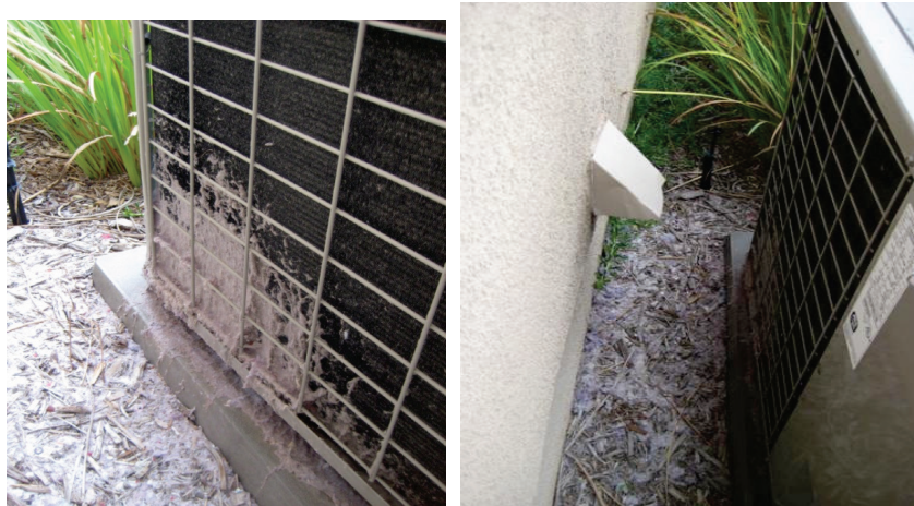
Figure 4-2: Noncompliant Condensing Unit Clearance From Dryer Vents
