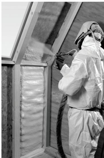
Figure 3-52: Closed-Cell SPF Installation in a Wall Cavity (full-fill not needed; thickness installed to achieve R-value only)
