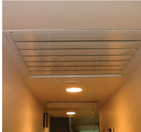
Figure 4-37: Whole-House Fan Damper
